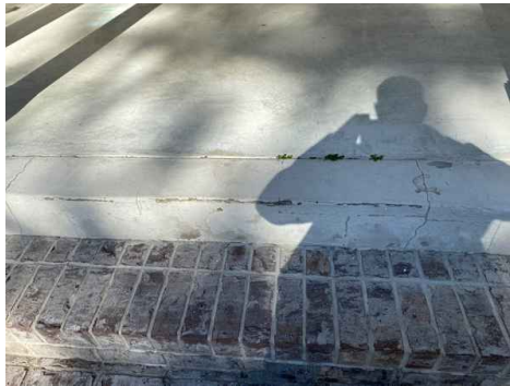
Minor cracking due to settlement
