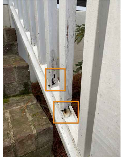
Wood Rot On Spindles
