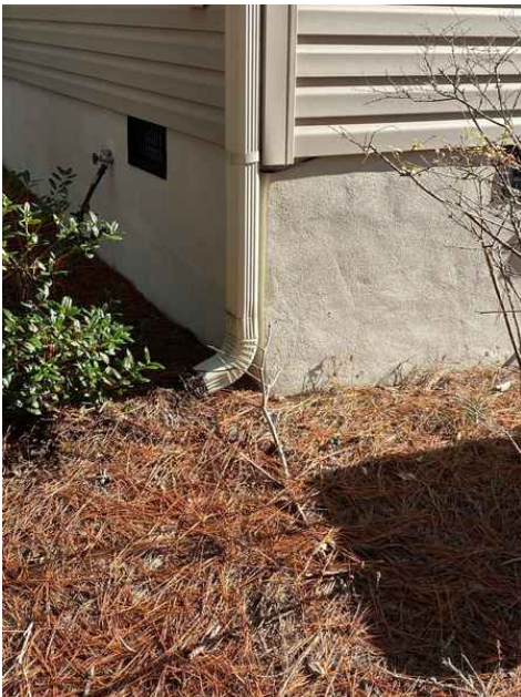
Left Rear downspout clogged with debris.
