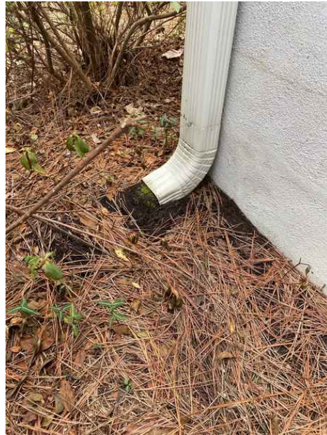
Rear, clogged with debris.
