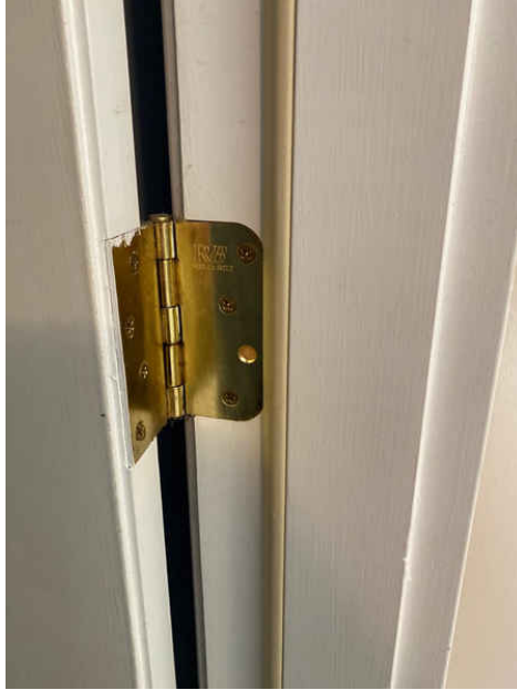
Garage Door Missing Screw
